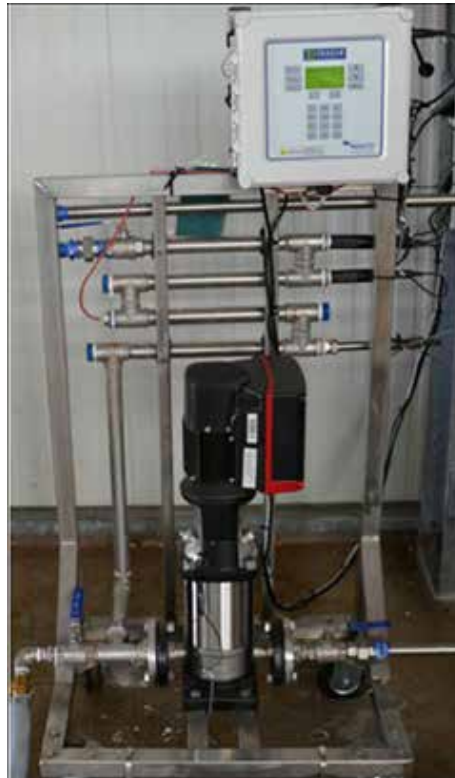
Figure 2: NCM skid for online corrosion monitoring.
