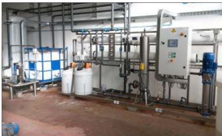
The new Nalco Water RO plant
